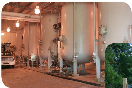
Large groundwater treatment system with five tanks of activated carbon.
