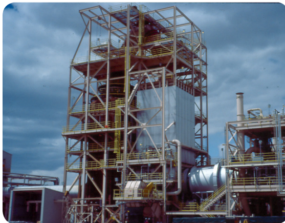
Example of offsite incinerator.
