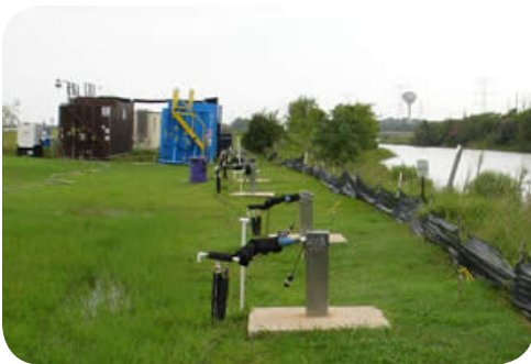
Groundwater Pumping Wells
