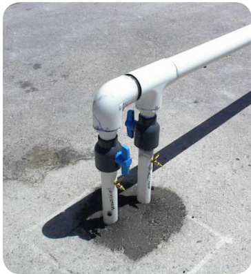
Pipes transport vapors from the underground SVE extraction well to treatment.
