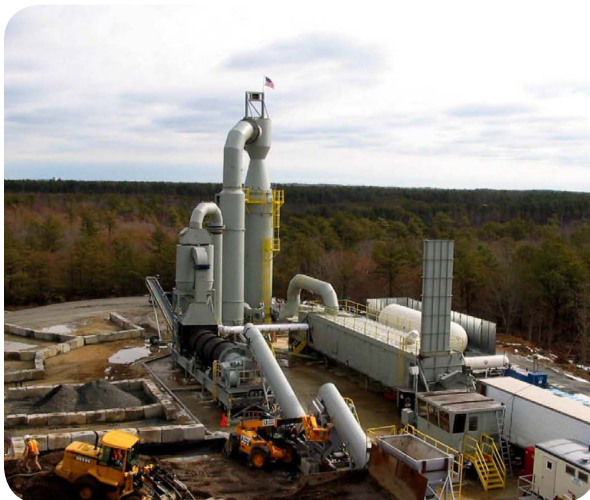
Onsite thermal desorber.
